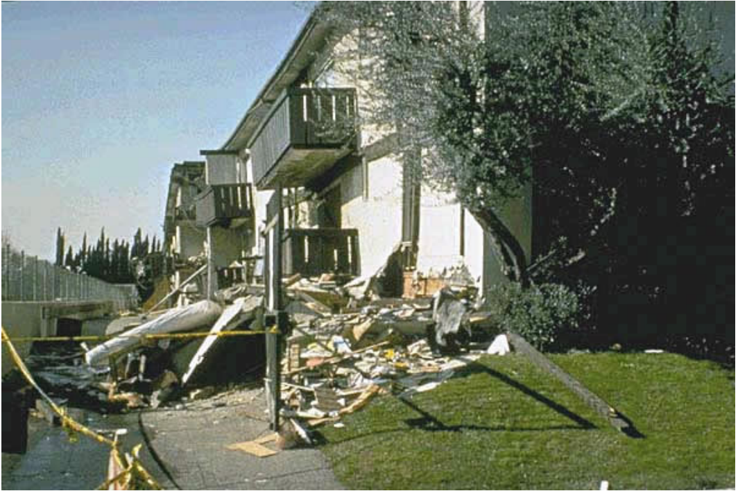
Figure 5-20. Collapsed first floor of Northridge Meadows Apartment.
