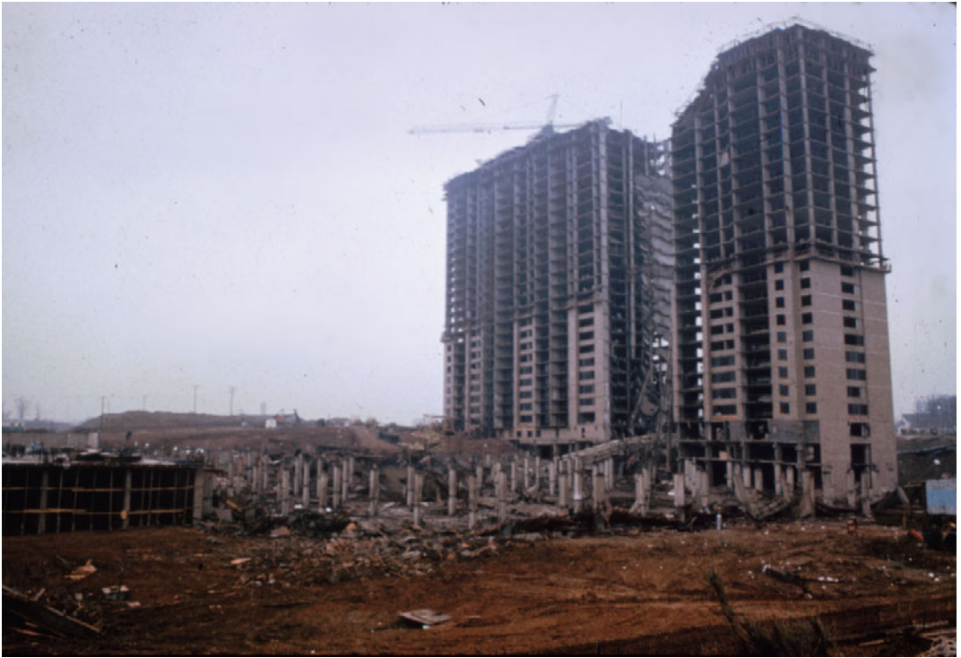
Figure 5-7. Overview of the Skyline Plaza Collapse at Bailey's Crossroads.
