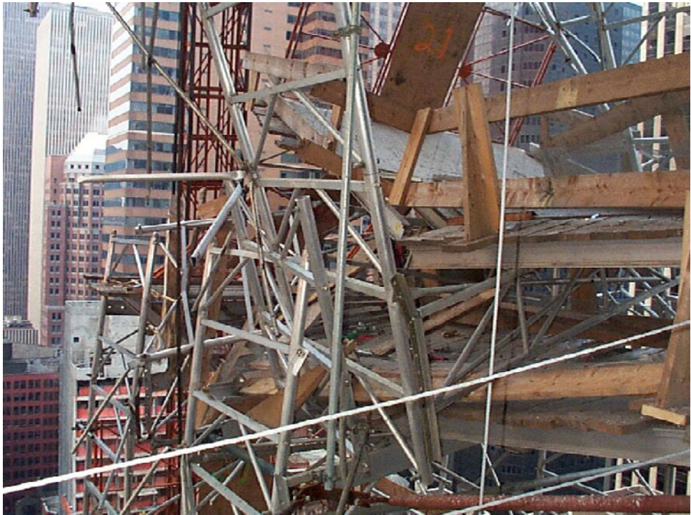
Figure 5-22. Collapse of scaffolding of Four Times Square.
