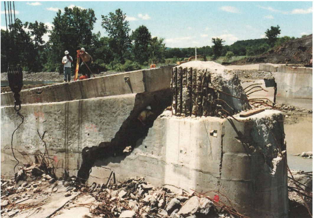
Figure 1-5. Schoharie Creek Bridge failed plinth.
