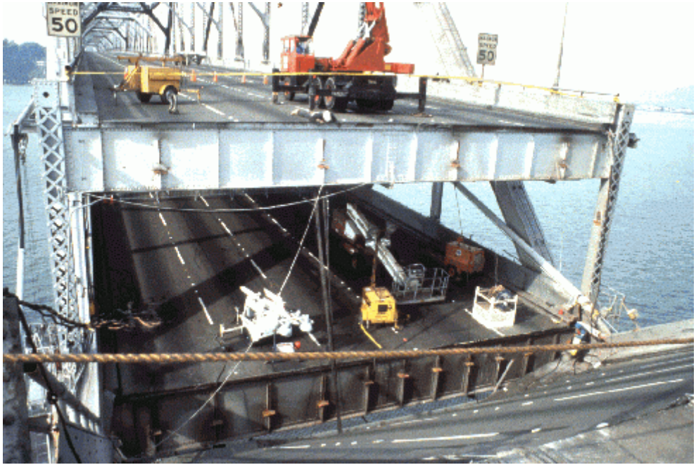
Figure 4-3. Damage to San Francisco-Oakland Bay Bridge.
