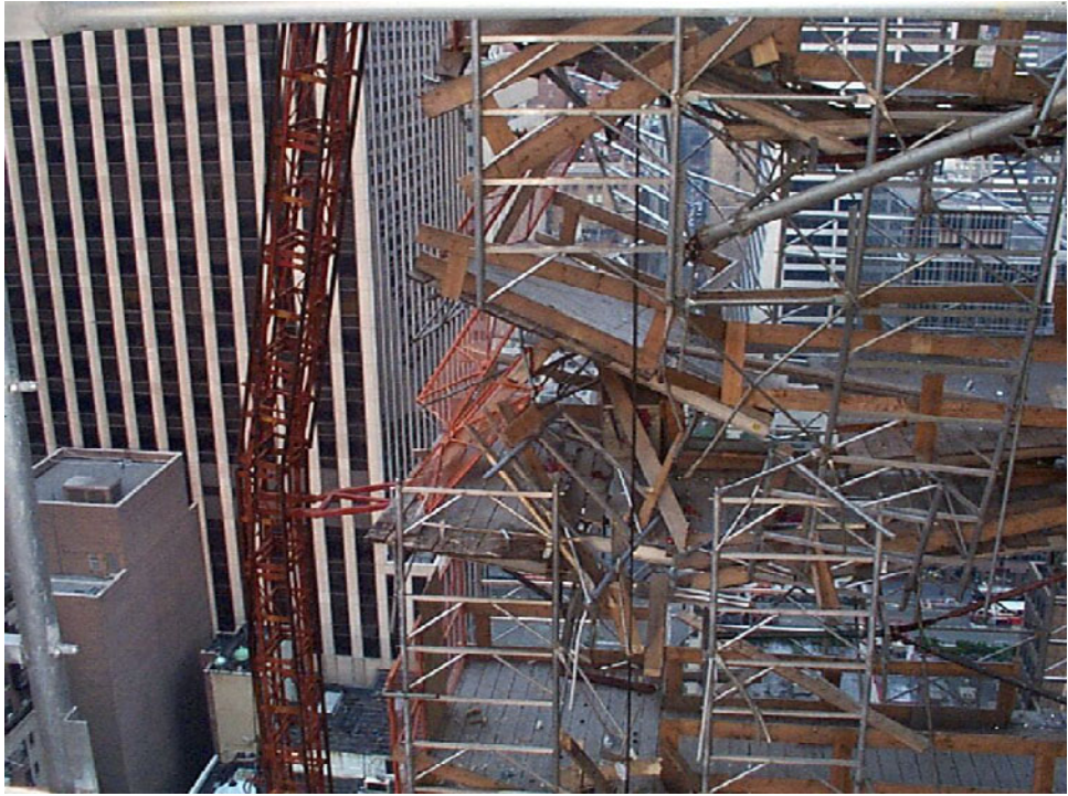
Figure 5-21. Collapse of scaffolding of Four Times Square.
