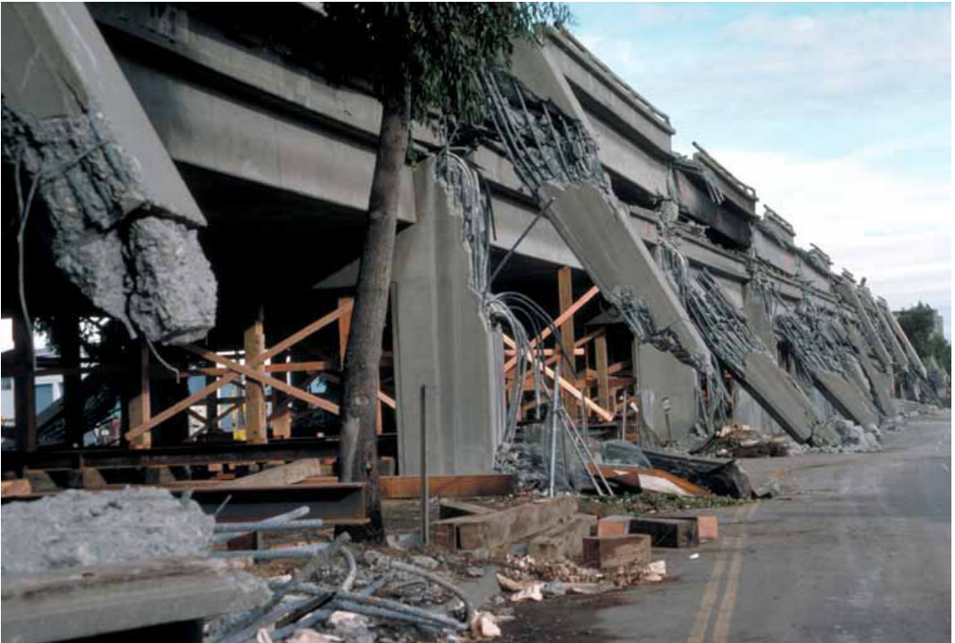
Figure 4-4. Cypress Viaduct Support Column Failure.
