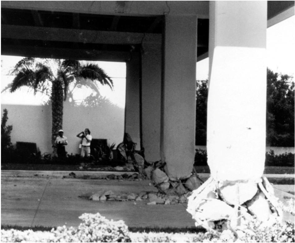
Figure 5-11. Column of Imperial County Services Building. Source: C.E. Johnson, USGS.
