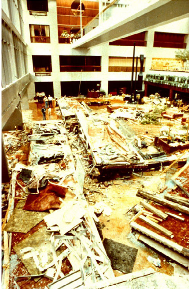
Figure 5-13. Second and Fourth Floor Skywalks collapsed in lobby. Source: Courtesy of Wiss, Janney, Elstner Associates, Inc.
