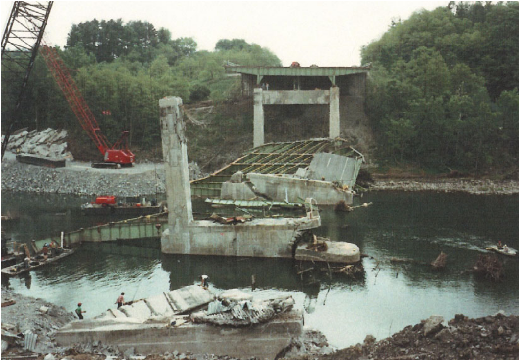
Figure 1-4. Schoharie Creek Bridge collapsed spans.
