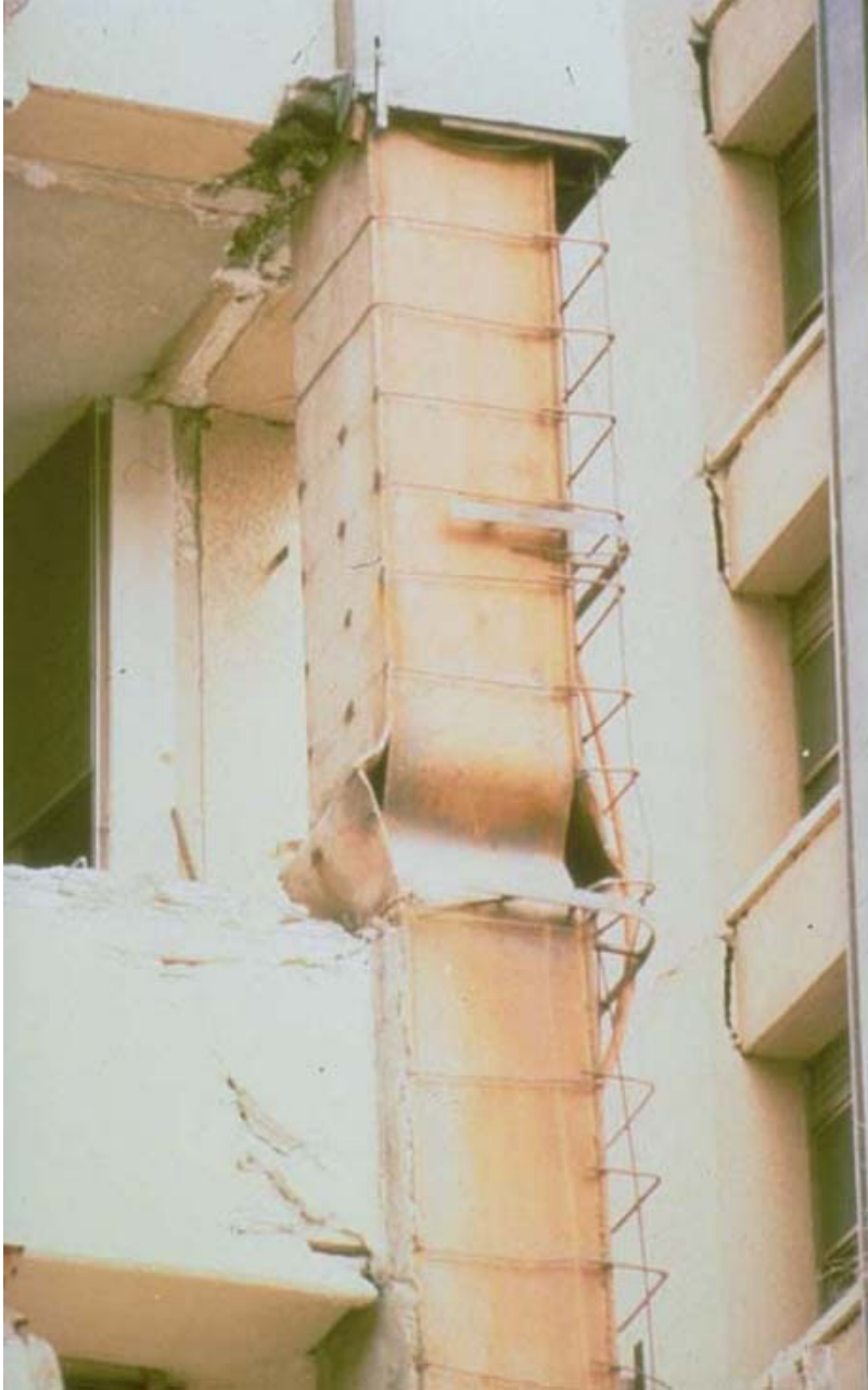
Figure 5-15. Pino Suarez Buckled Column.
