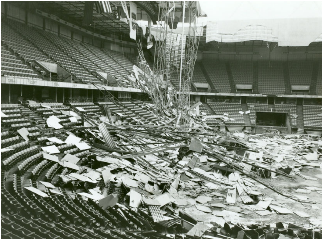
Figure 5-12. Kemper roof debris litters seats below shortly after the collapse.
